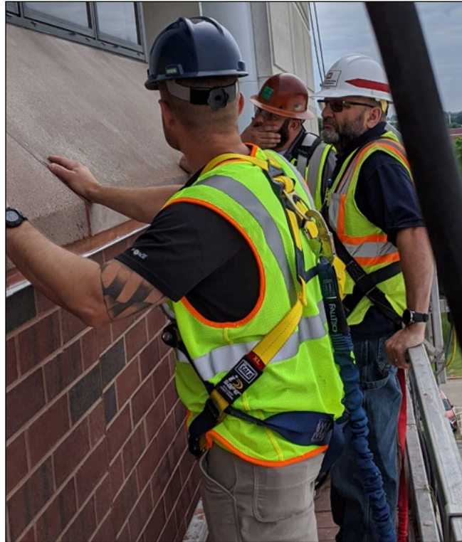
Todd Decosse (middle), St. Paul District construction representative, and two contractors, work on the Minneapolis VA Medical Center in Minneapolis, June 23, 2020. USACE courtesy photo
