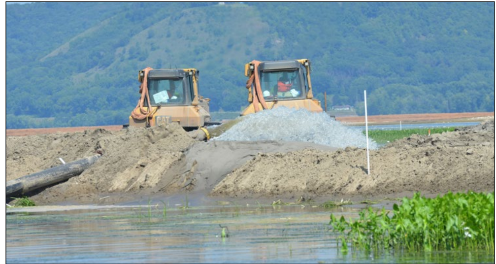
Work being completed on Capoli Slough Islands restoration project, near Ferryville, Wisconsin, Aug. 23, 2013. USACE photo by Patrick Moes
