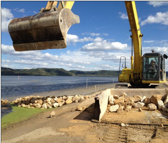
Corps employees complete construction on Capoli Slough Islands restoration project, near Ferryville, Wisconsin, Sept. 20, 2012. USACE courtesy photo
